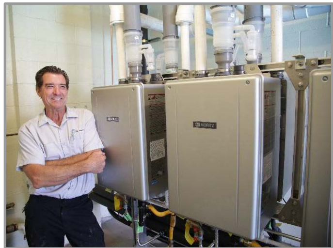
James Motis, owner of Prevent Backflow Plumbing, stands in front of the Noritz NCC199CDV multi-unit system he installed at Mater Dei High School.
