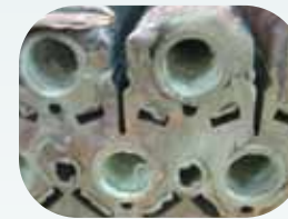
Scale build-up on a Norritz heat exchanger in an extremely hard water area.
