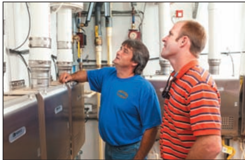
Installer Anthony Crouch (left) with Jason Veal, who describes the 17-unit tankless installation at the Florence Residence Inn as “a positive experience for everyone involved.”
